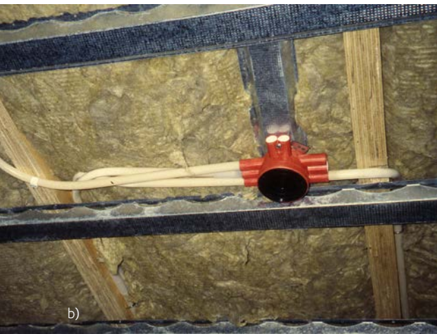
Figure 8.19 a) Typical floor design in timber frame building system. b) Photo of the bottom part of the floor with electric installations.
